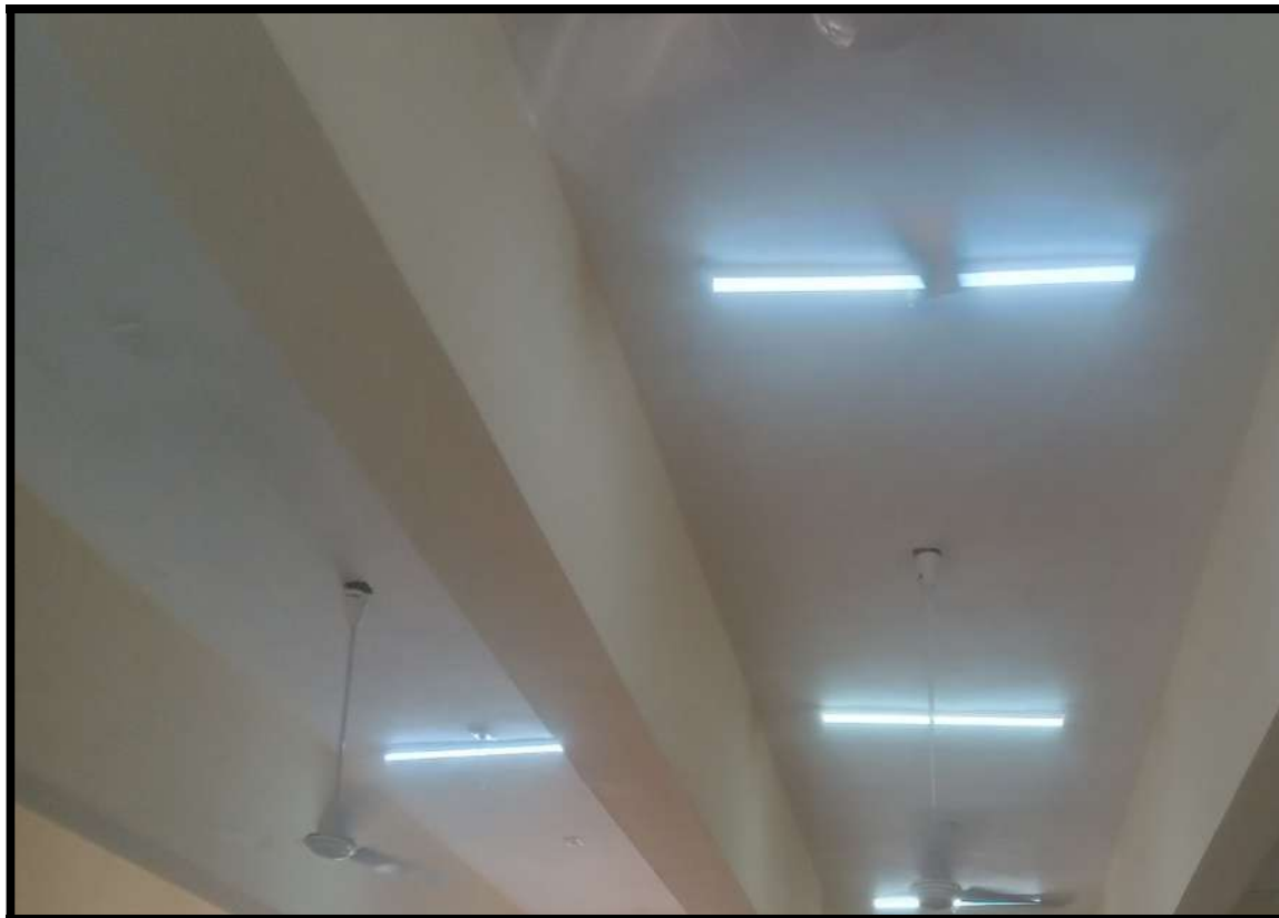
ENERGY EFFICIENT LED LIGHTING FIXTURES & CEILING FANS
