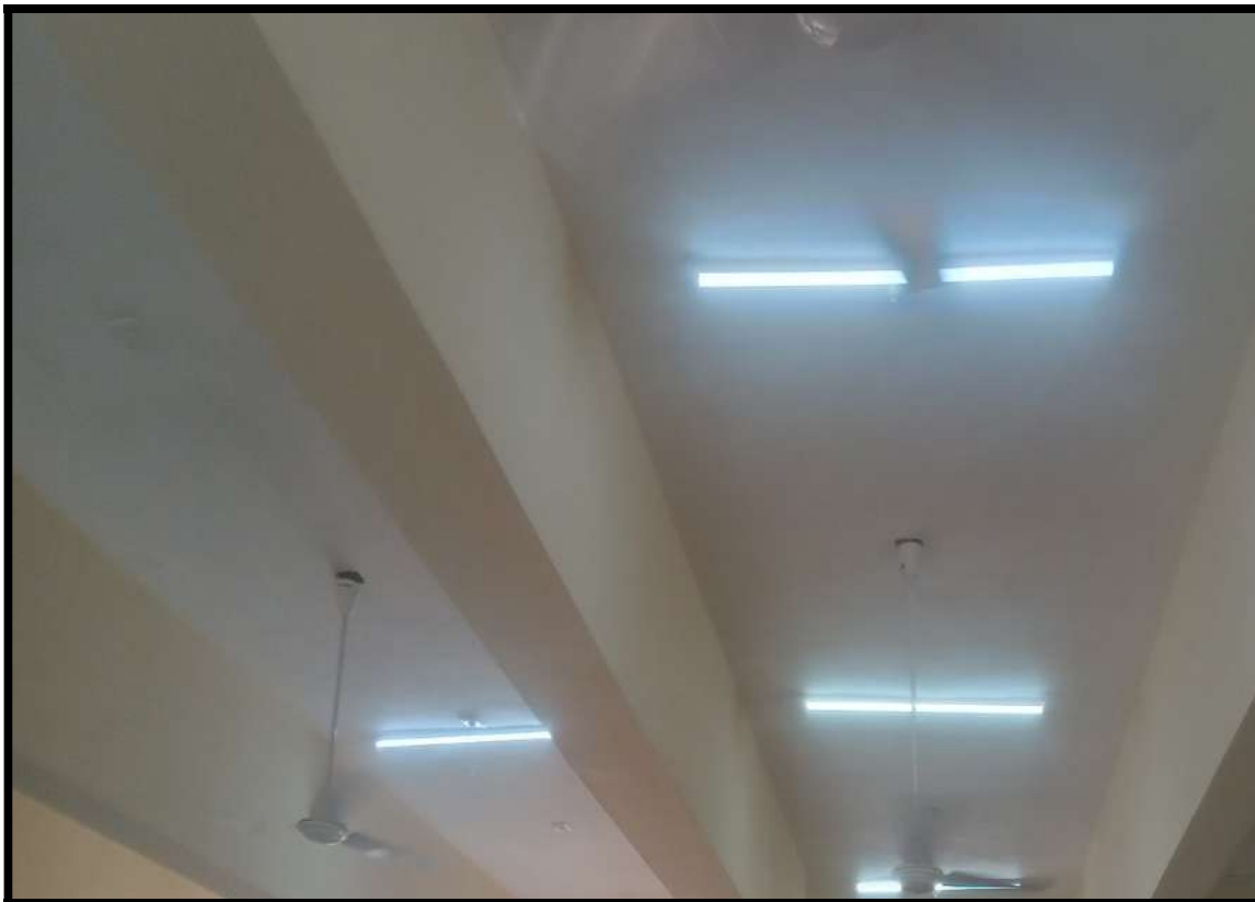
ENERGY EFFICIENT LED LIGHTING FIXTURES & CEILING FANS
