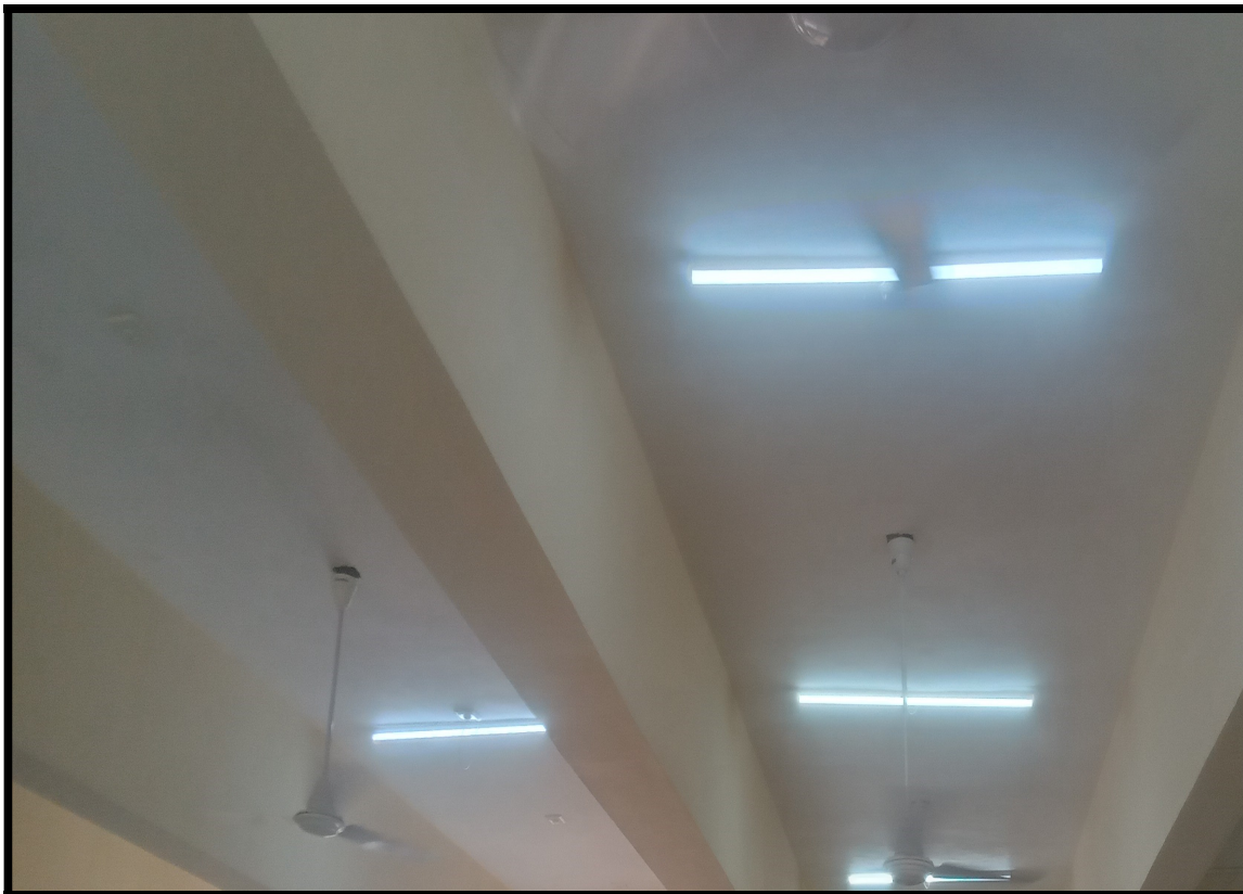
ENERGY EFFICIENT LED LIGHTING FIXTURES & CEILING FANS
