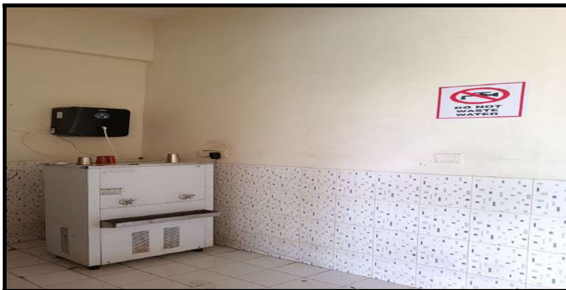
WATER COLLER WITH FILTRATION FACILITY
